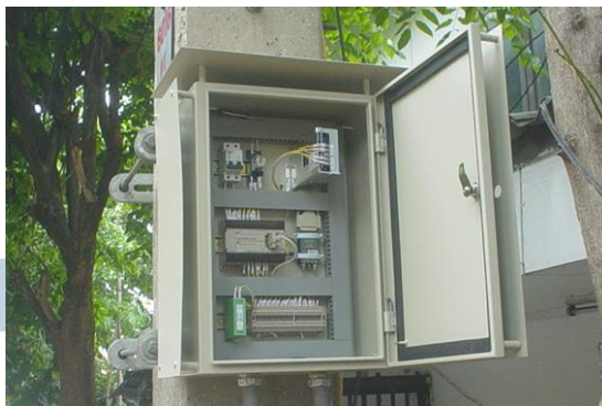
Fig. 7. Cubicle of Remote I/O Device
